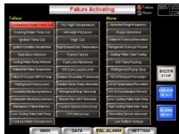
Failure & Alarm screen
